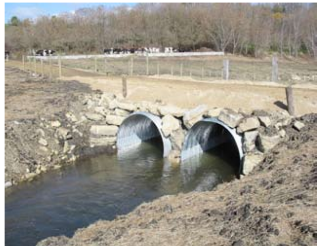
Note the change in water height within the culverts which allows for fish migration.
