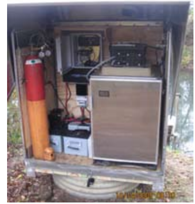
USGS gaging station showing automated water-quality sampler and monitoring equipment.
