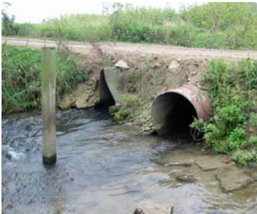
Perched culverts before installation of replacement culverts.
